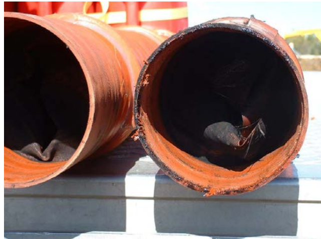
Figure 7.3-2 Delaminated Exhaust Tubing
