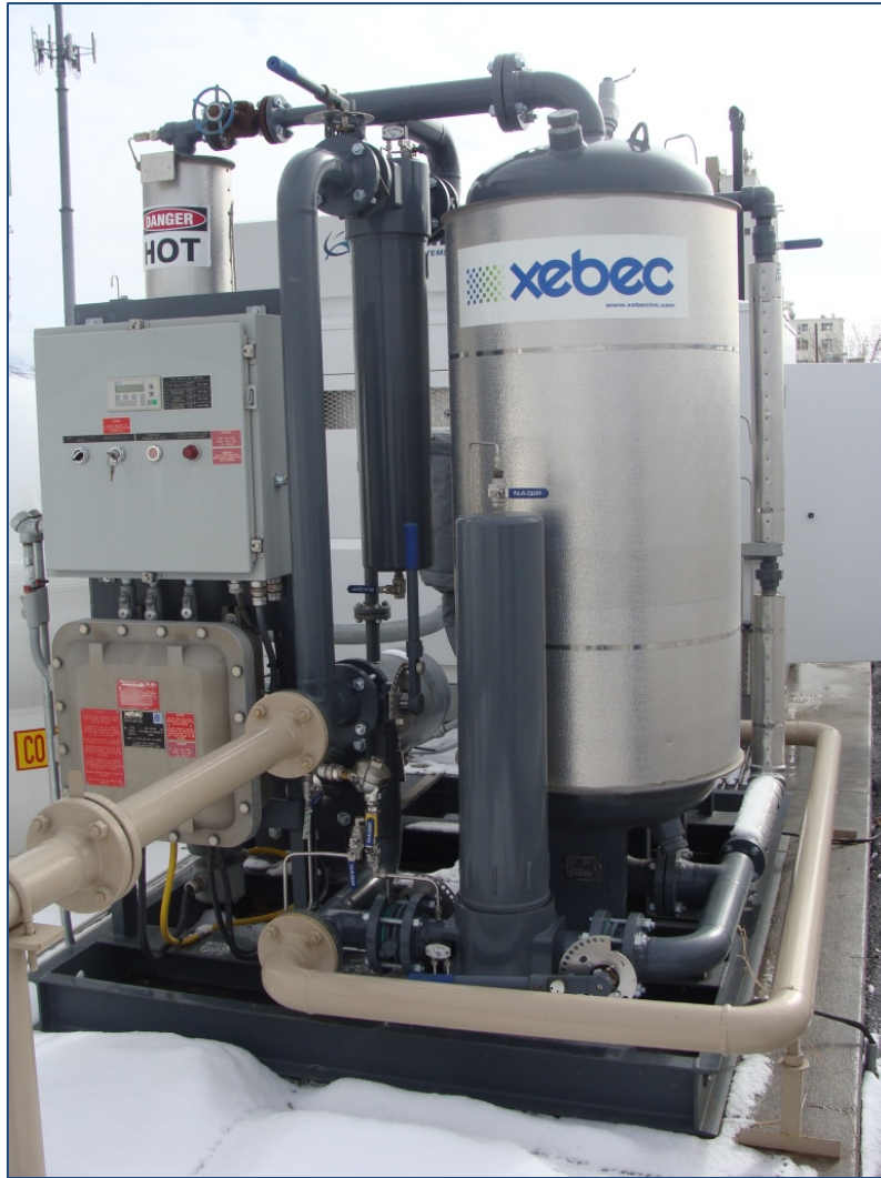
Figure E.20. Dehydration Skid at Station W4
