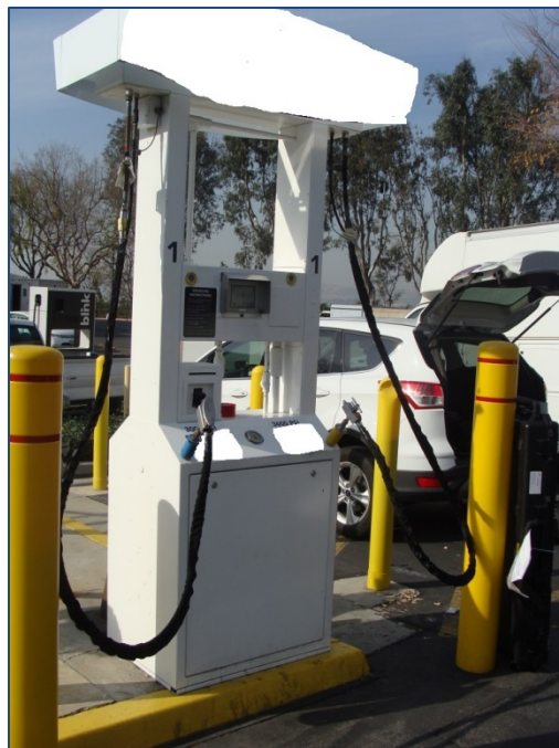
Figure E.17. Dispenser at Station W3
