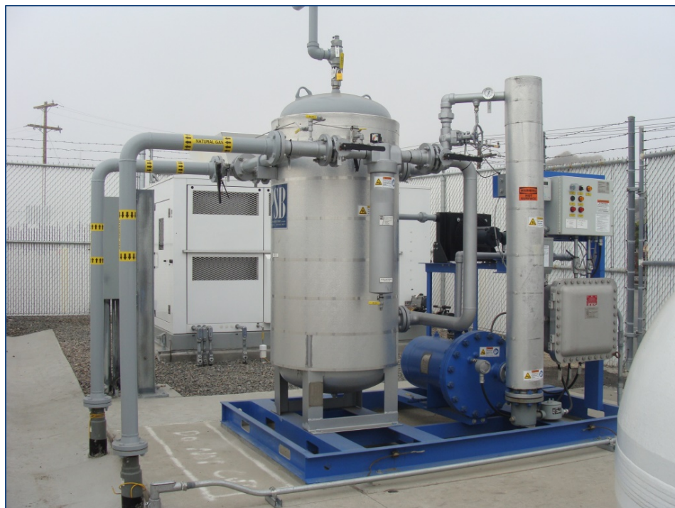
Figure E.9. Drying Skid at Station W2 The tall cylinder toward the right is the desiccant stack where drying occurs. Dry gas passes through the receiving tank and filter in the center of the photo on its way to the compressors (in the white structure behind the drying skid).
