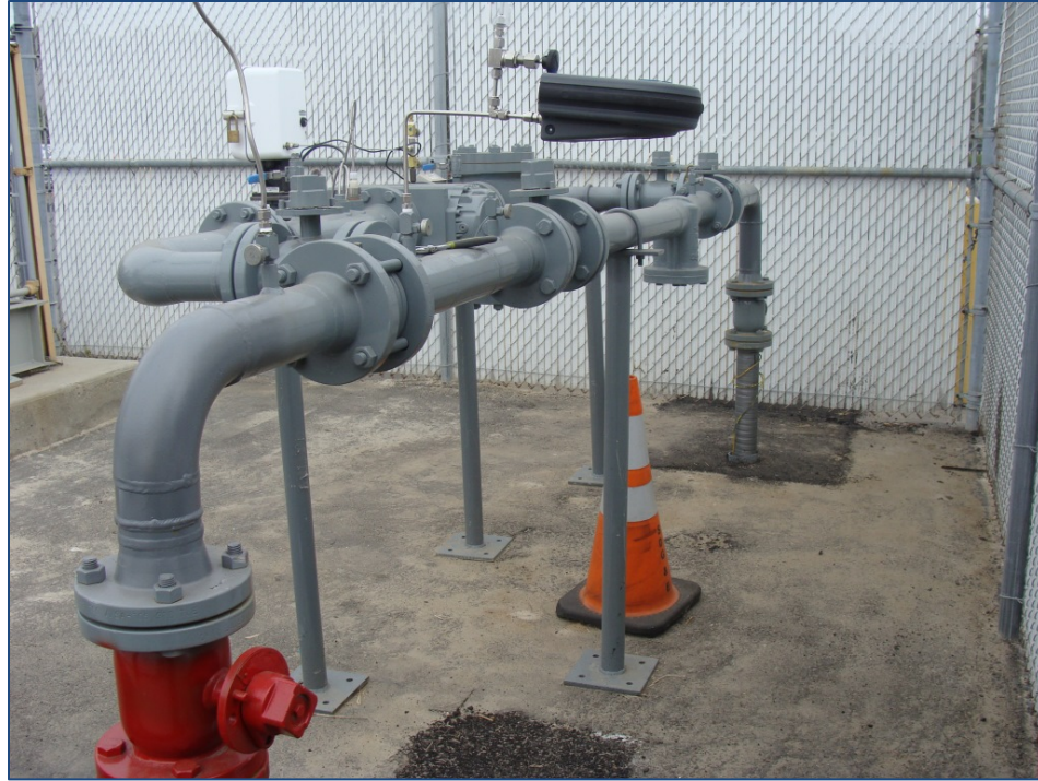
Figure E.8. LDC Custody Transfer Meter Run at Station W2 Moisture measurements of the incoming gas were taken from a sample tap downstream of the rotary meter used for custody transfer.
