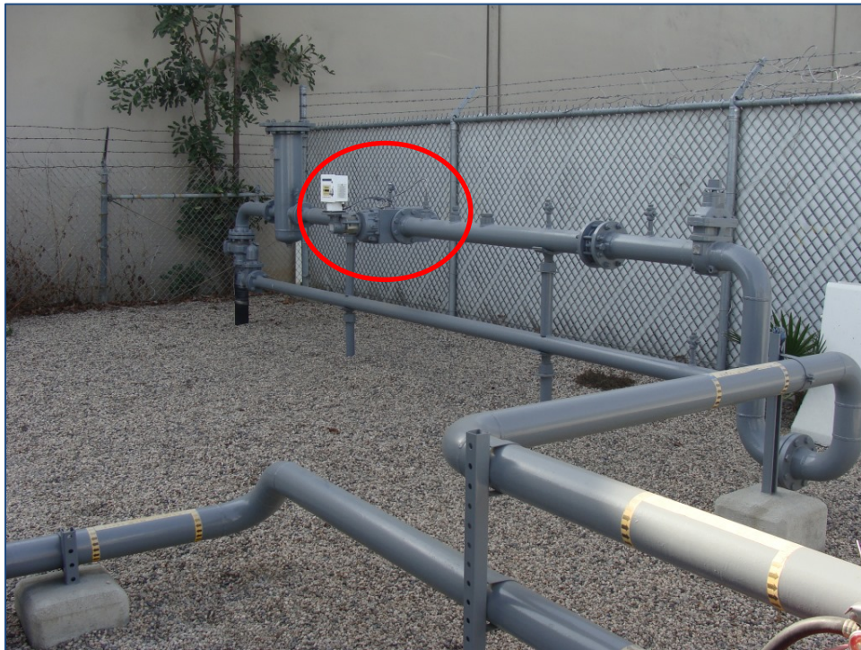
Figure E.2. LDC Custody Transfer Meter Run at Station W1
