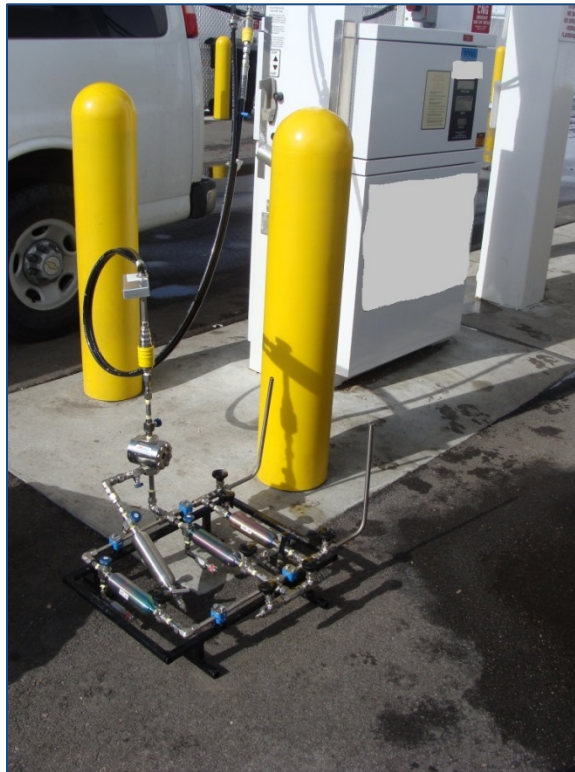
Figure E.22. Dispenser at Station W4
