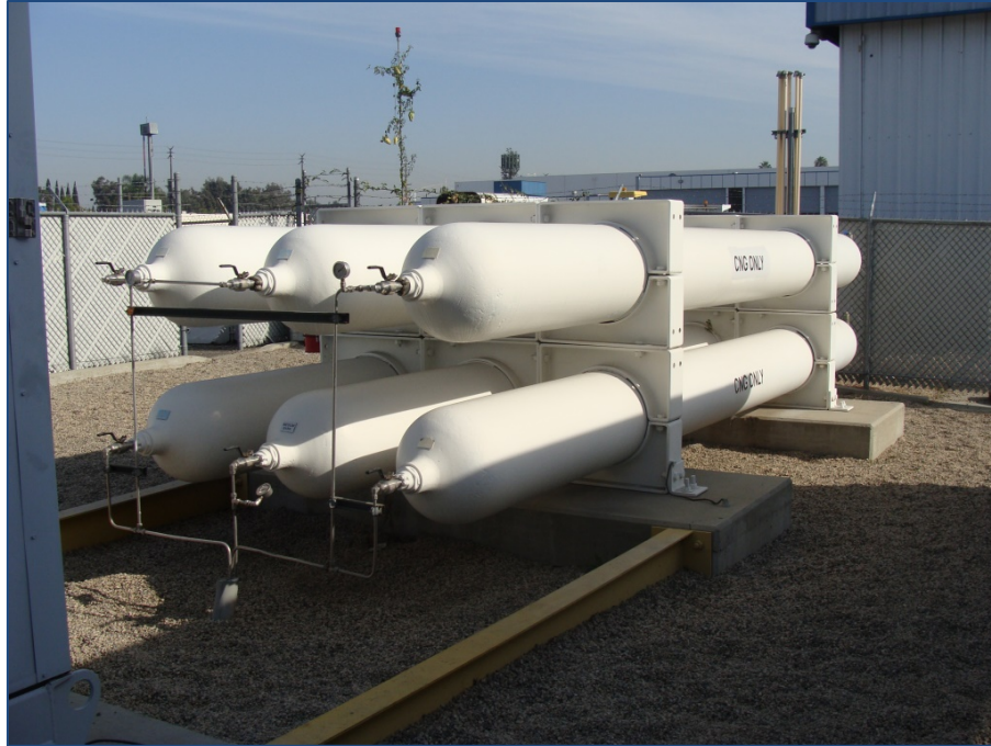
Figure E.5. CNG Storage Tanks at Station W1
