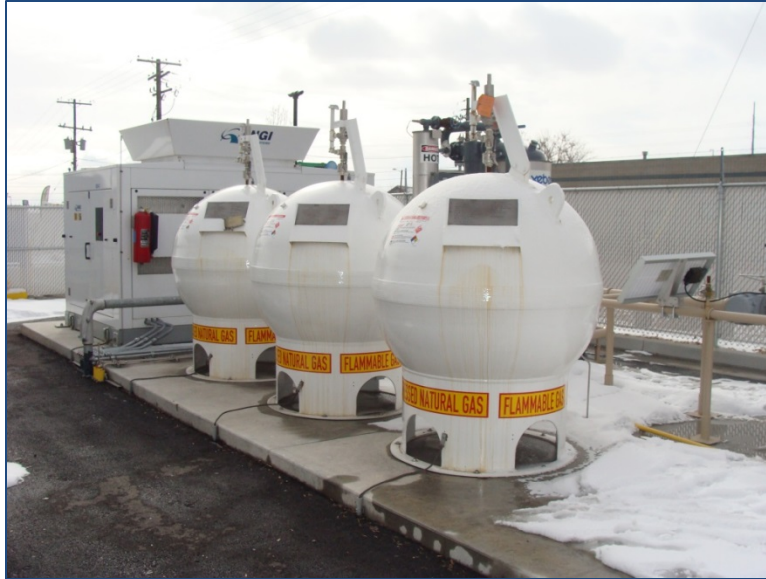
Figure E.21. Compressor Skid and CNG Storage Tanks at Station W4
