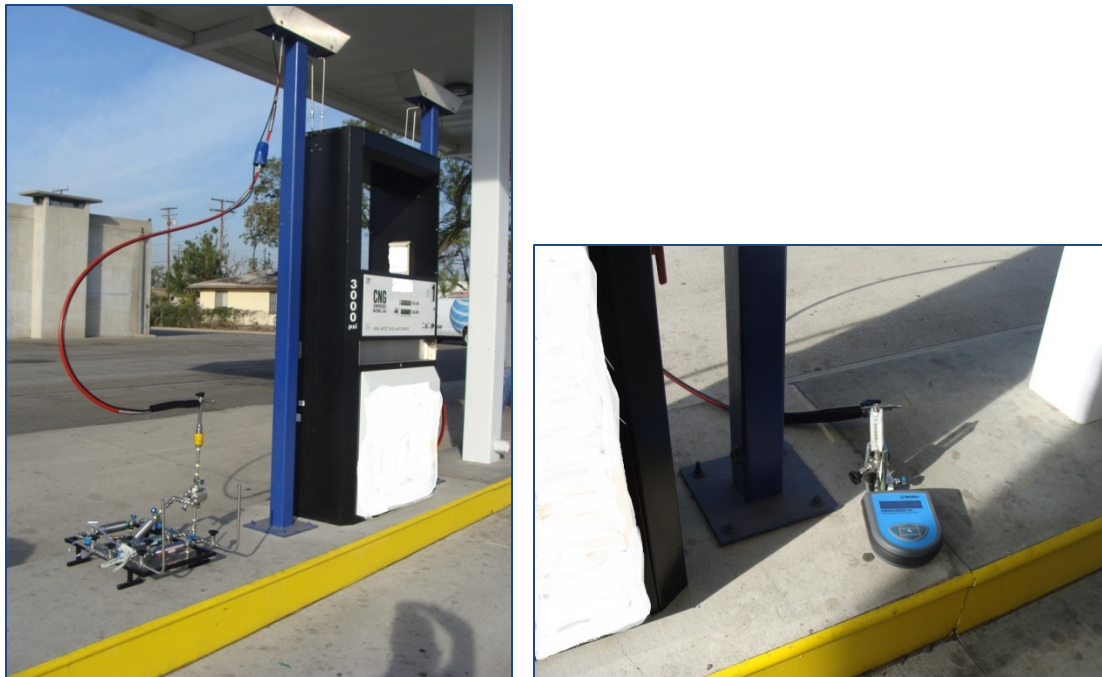
Figure E.6. Dispenser at Station W1
