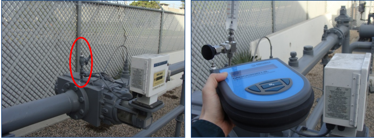
Figure E.3. Moisture Measurement Location at the W1 LDC Connection
