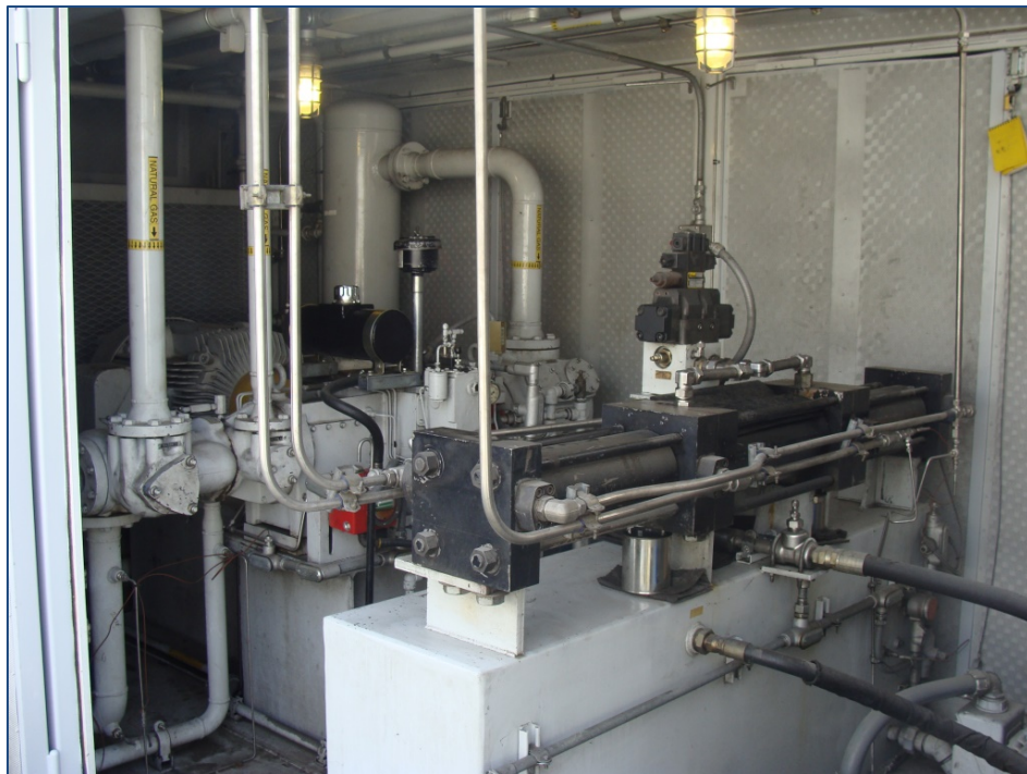
Figure E.15. Interior of the Drying and Compression Skid at Station W3 All drying, compression, and filtration equipment at this station is enclosed in a prefabricated skid. Parts of the compressor can be seen in the foreground and at the left rear. The desiccant stack is behind the wall at the left rear of the photo.
