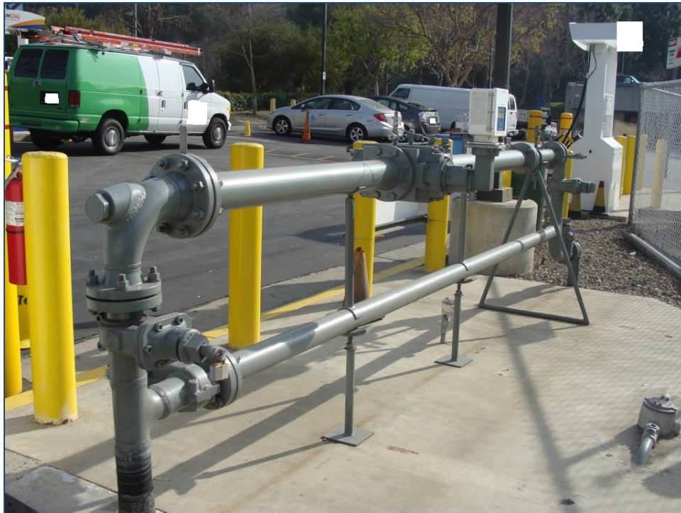
Figure E.13. LDC Custody Transfer Meter Run at Station W3
