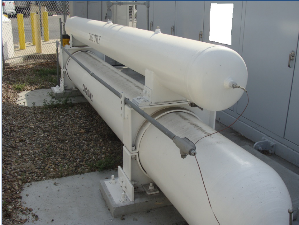
Figure E.16. CNG Storage Tanks at Station W3
