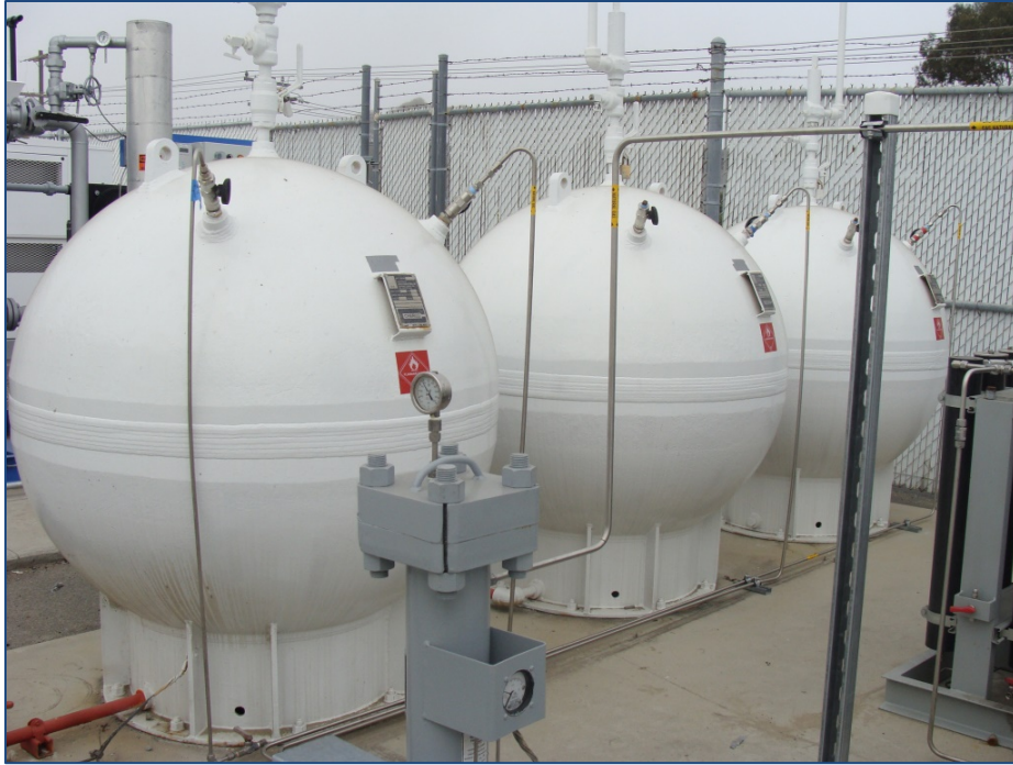
Figure E.10. CNG Storage Tanks at Station W2 Unlike most CNG stations, station W2 uses spherical CNG storage tanks.
